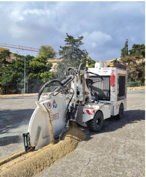
Fiber optic & Telecom
